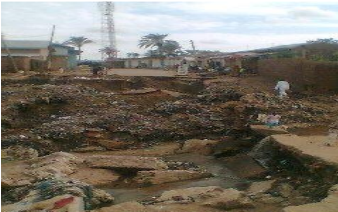
Plate 2. Bello Sabo Kudi road/ bridge destroyed by flooding in 2004. Source. Field work, 2011
